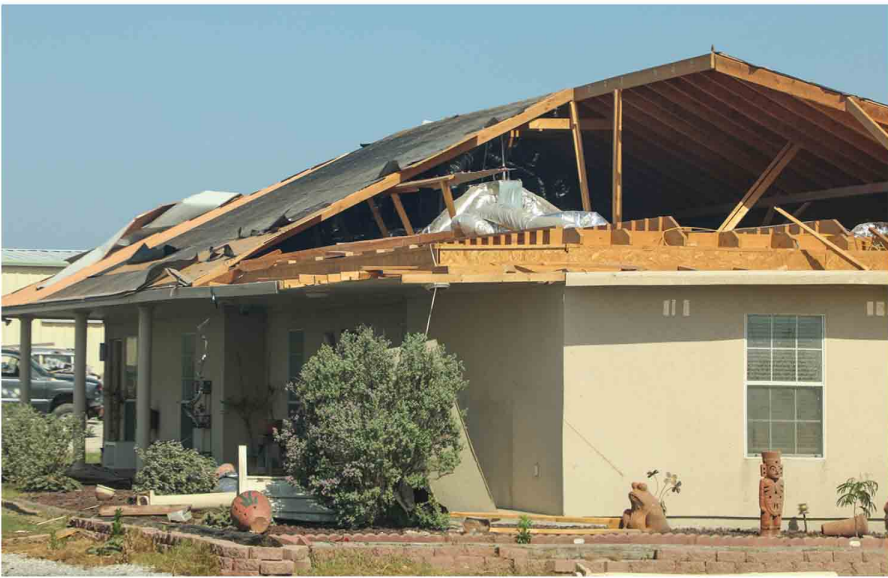
Fish n Hook Boat Storage (home/office) off of FM 455E is damaged.
