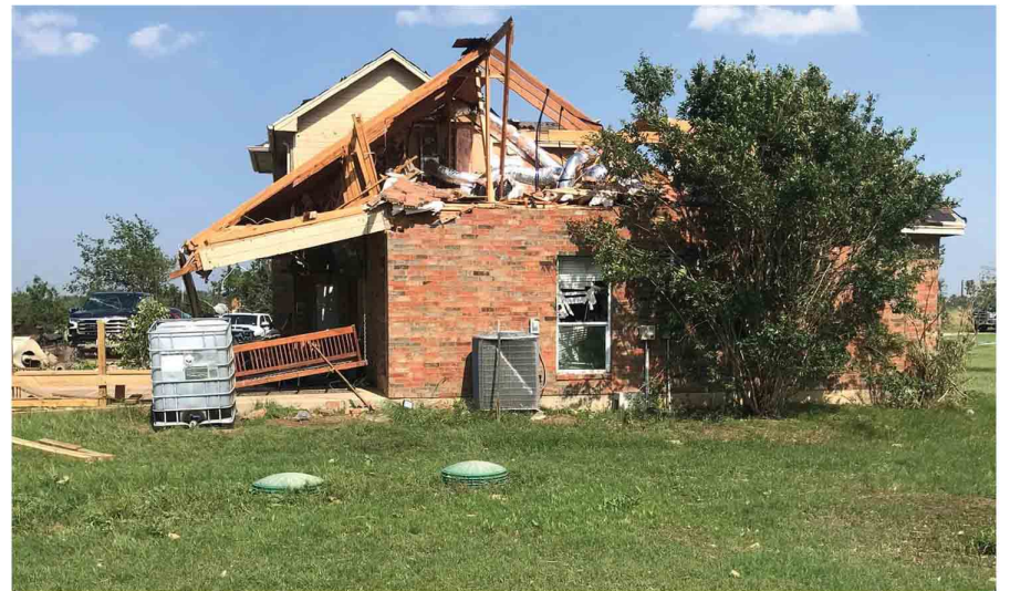
A home off Chisam Road, near Huling Road has severe damage.
