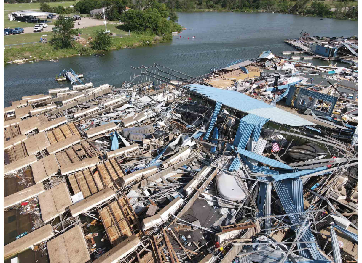
Boat houses one and two (hundreds of slips) at the Lake Ray Roberts Marina, just east of Sanger off FM 455, the gas dock/ships store were flipped upside down or mangled from the tornado.
