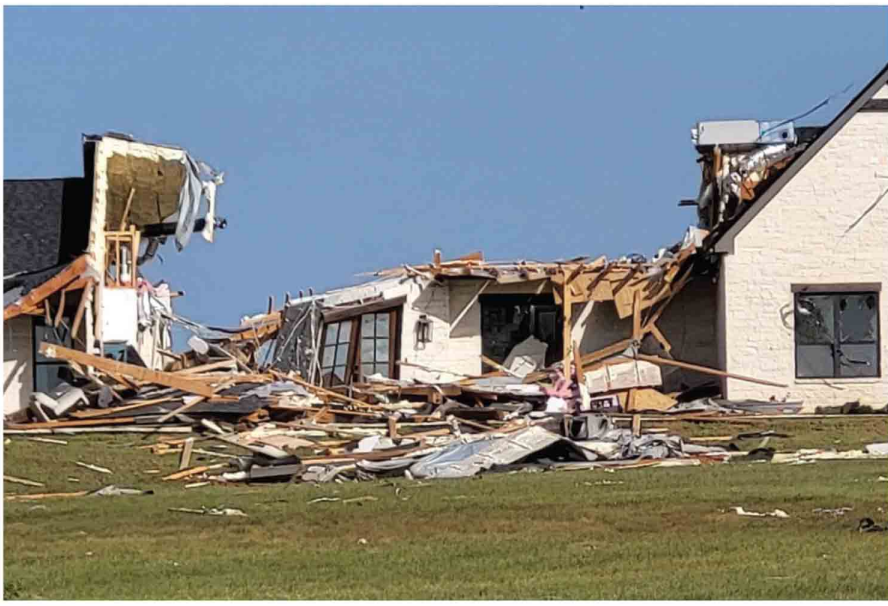
A new home near the local marina and Jones Road took a direct hit from the tornado.
