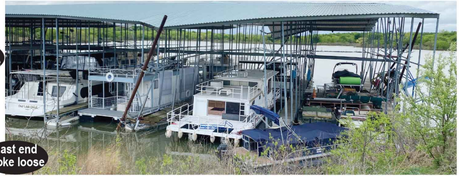
Boat house 9 brace poles (pipes) are tilted over from the high winds.
